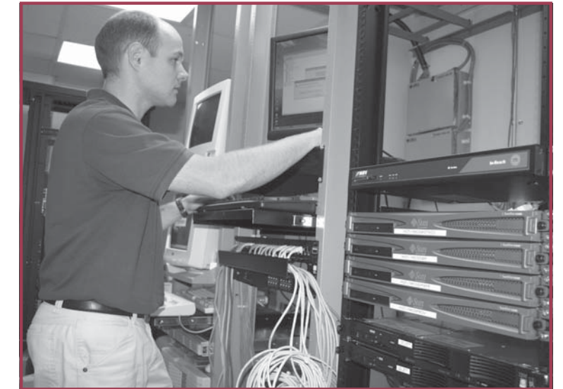
Adam Wagner from Softek doing HGT network conversions for the Nortel MCS 5100 install at Saint Vincent Health System
