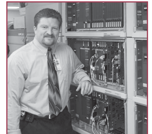
HGT's Jeff Scarpitti with the new Nortel Switch located at Saint Vincent Health System
